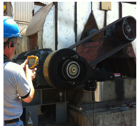
A Flux Drive Technician uses instrumentation to confirm overall alignment and vibration levels.
