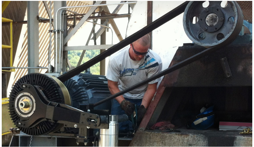
Flux Drive Adjustable Speed Drive installation on the 200hp ID Boiler Fan
